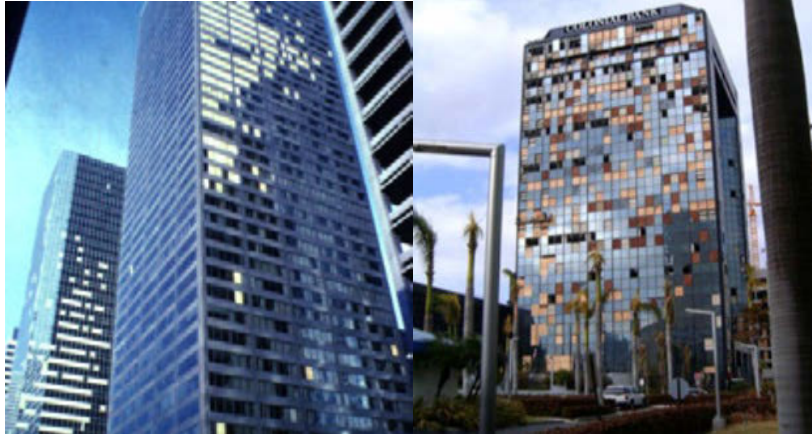
Figure 1. Building Damages during Hurricane Alicia in 1982 (left) and Hurricane Wilma in 2003 (right), by Beers [1]
